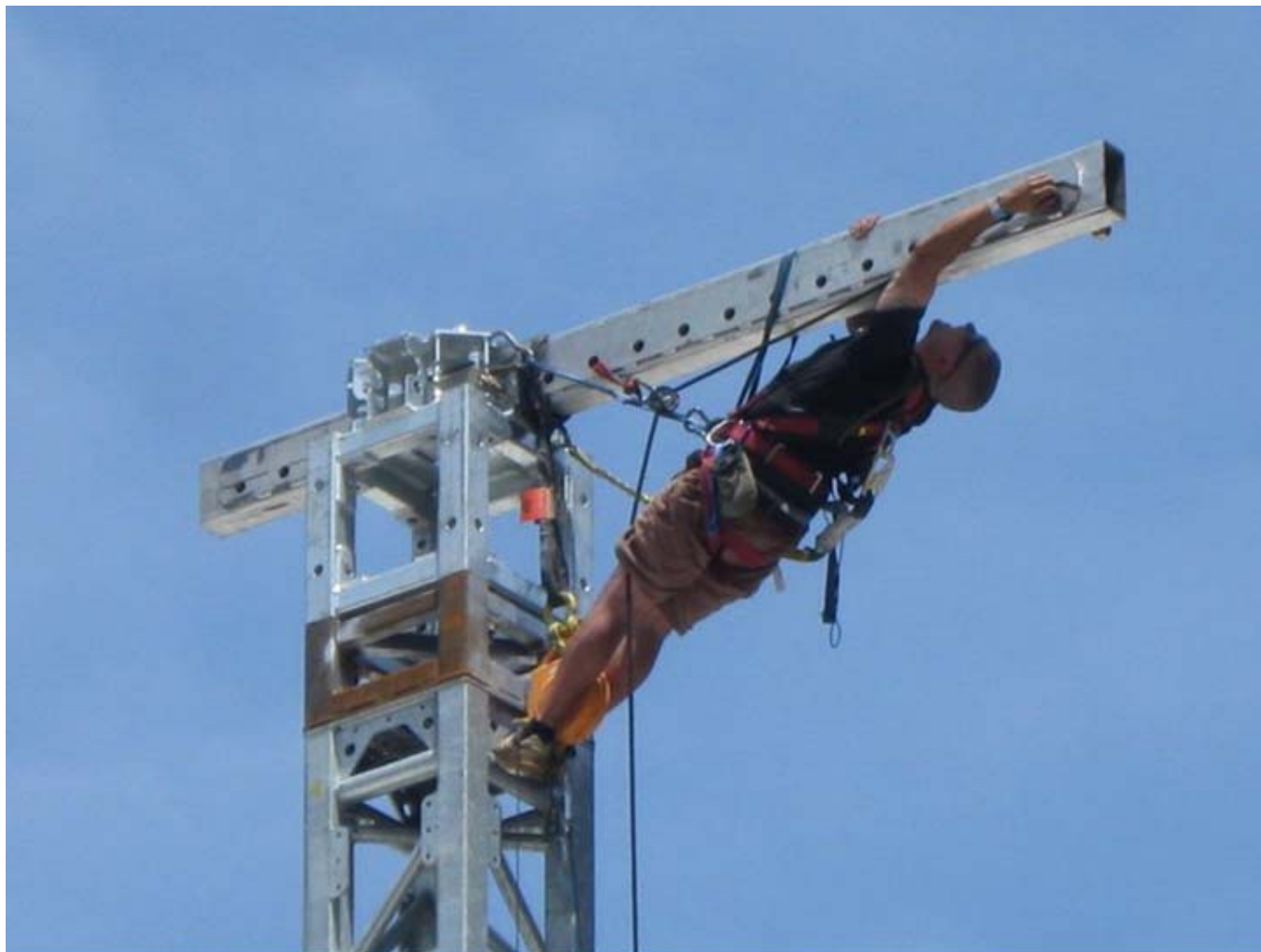
Local No.4 Member, Daniel Nieves, 50 feet up prepping a roof tower for The Dave Matthew's Band, Citifield 2010
